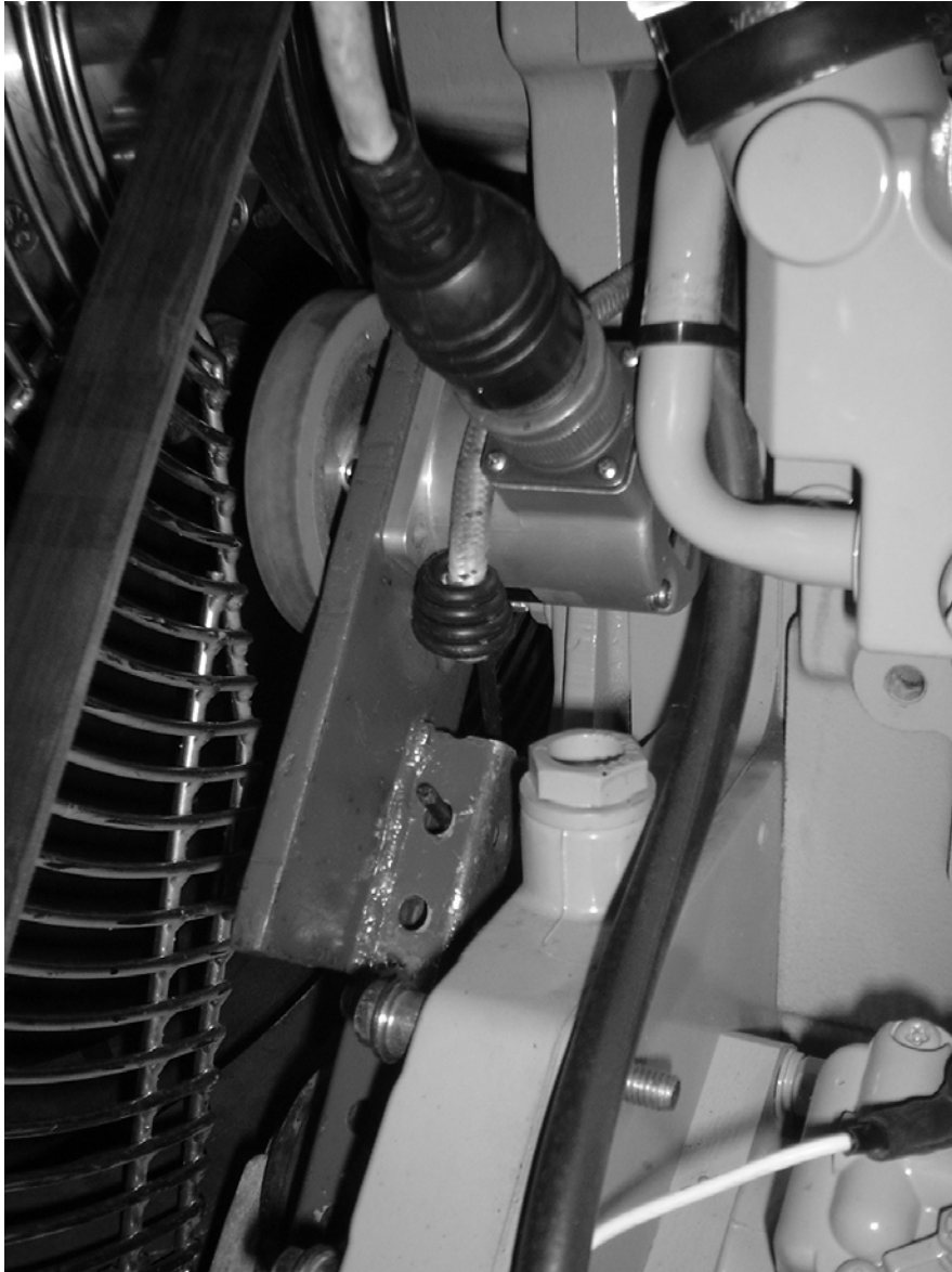
Figure 51 – Optical Encoder Mounting on Fan Drive Sheave
